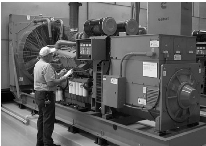
A well-planned maintenance program is essential to the operation of any power generation system.
